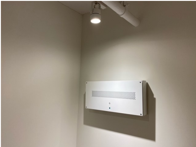
Leaf installation in private offices Return to work with a healthy mindset
