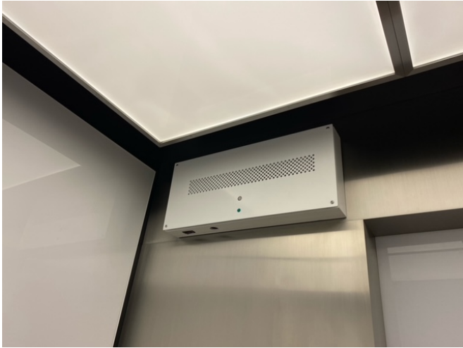
Leaf installation in elevator cabs Always assuring healthy air quality
